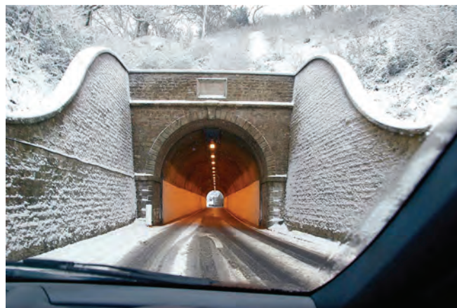
A view from inside the Beaminster Tunnel, looking south. Note the narrow carriageway and high roof. Photo Wendy Chatterton
